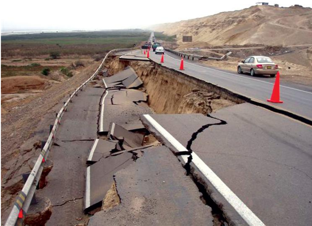
Figure 2.2. Highway Embankment Failure ( http://mceer.buffalo.edu )
