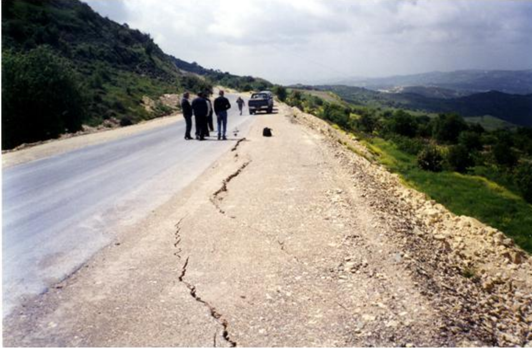
Figure 2.1. Evidence of Embankment Slope Deformation ( http://mceer.buffalo.edu )
