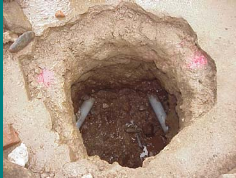
3 conduits interfere with 36" pole footing diameter
