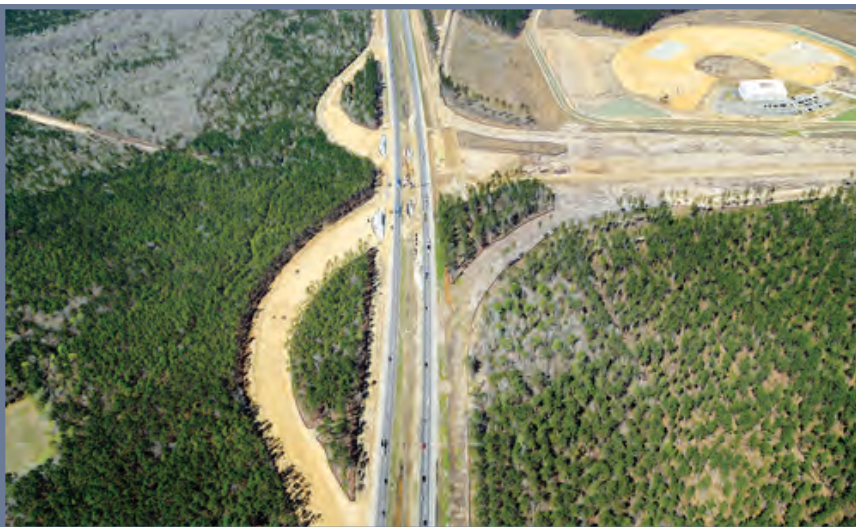
The ramps are taking shape as work continues on the Volvo Interchange.
