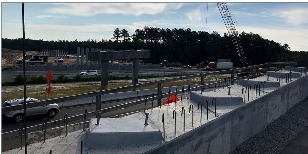
Left Image: Piers in place ready for bridge girders over I-26 Eastbound.
