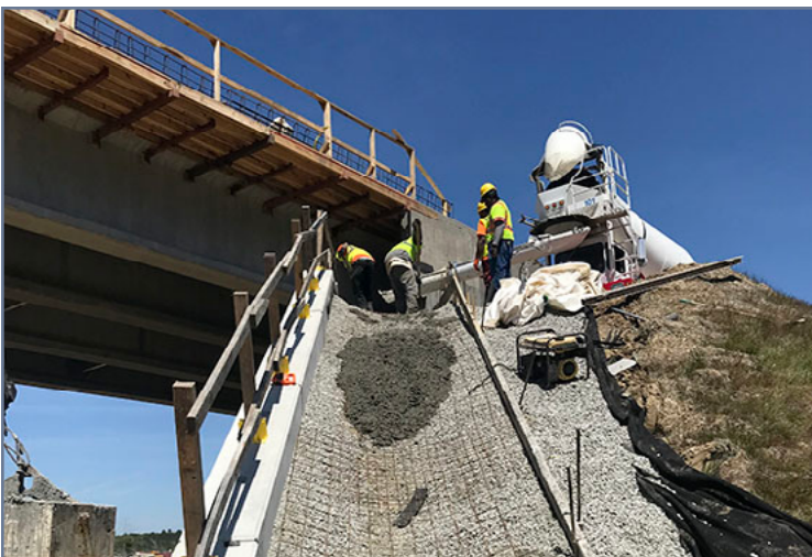
The Volvo Interchange crew installs concrete flumes on slopes to aid in channeling stormwater.
